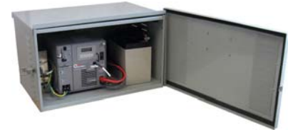
SSP-12 installed in CSEP1-120 enclosure
