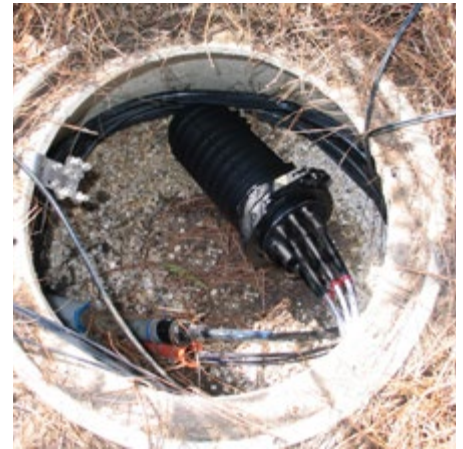
Hand Hole / Below Grade
